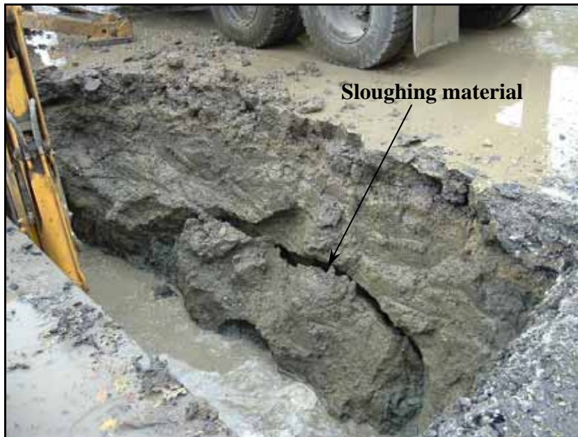
Figure 7. Material sloughing off the edges of the trench
