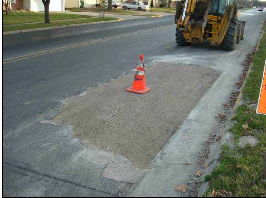
Figure 30. Utility cut left open for two weeks
