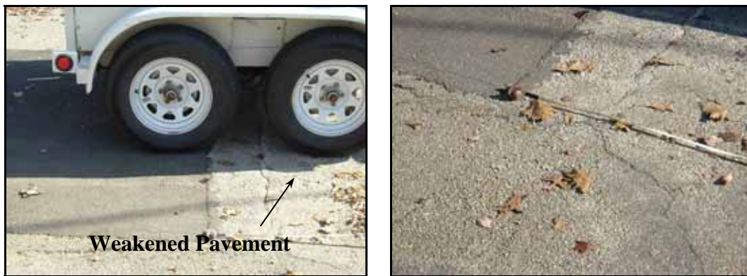
Figure 63. Cedar Rapids pavement distress
