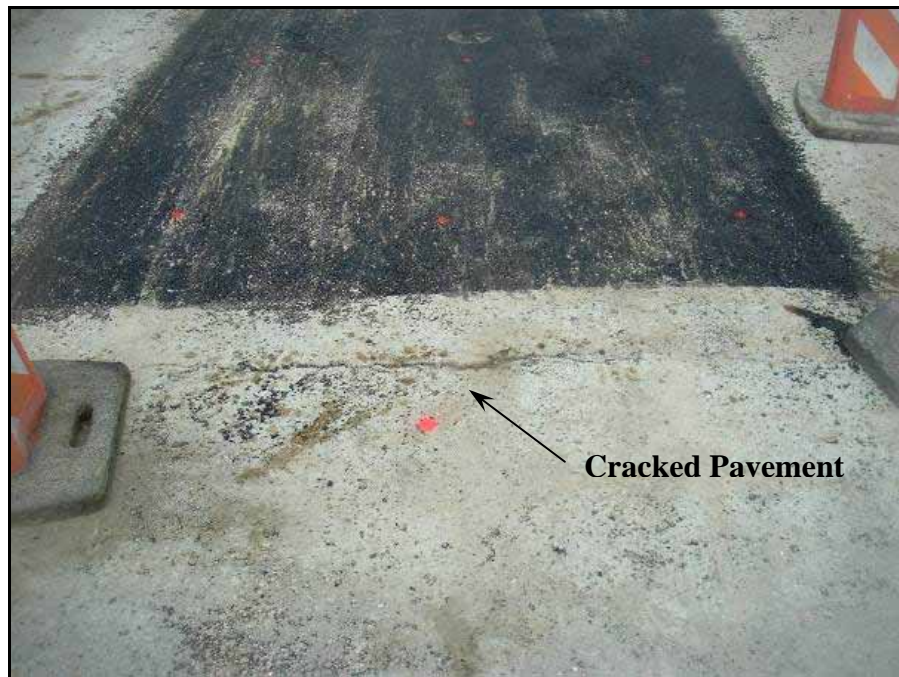
Figure 42. Visible pavement damage on utility edge
