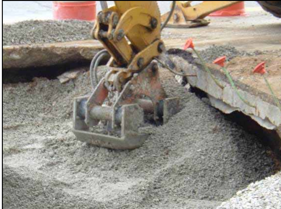
Figure 44. Large cavities forming beneath pavement
