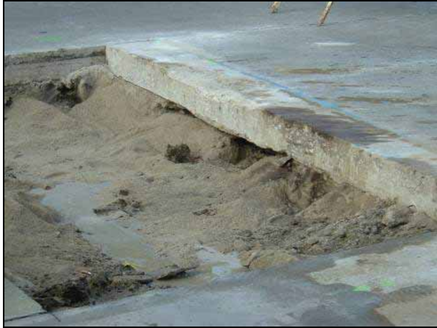
Figure 45. Backfill material caving in on trench edges
