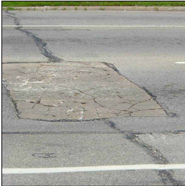
Figure 5. Temporary cold patch in Cedar Rapids, with an estimated age of three years
