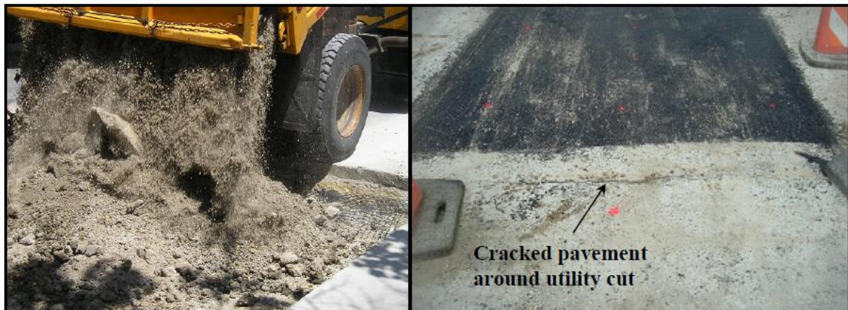
Figure 9D-1.01: Cracking Pavement Surrounding the Utility Cut Area Because of Construction Equipment Getting Too Close to the Edge of the Open Cut
