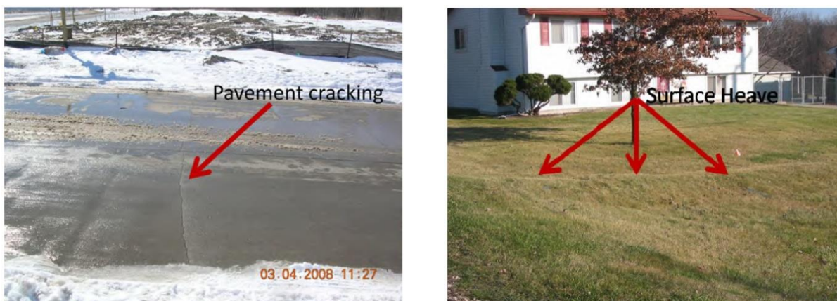
Figure 14B-2.07: Pavement Cracking Caused by HDD Installation
