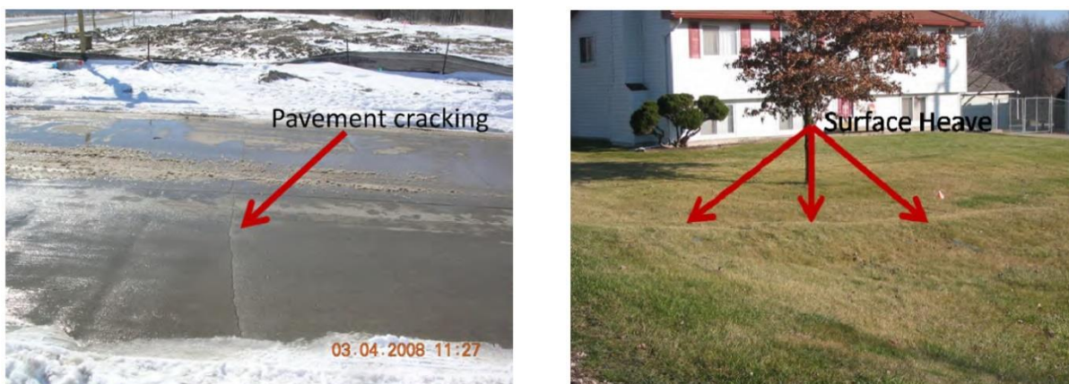
Figure 14B-2.07: Pavement Cracking Caused by HDD Installation
